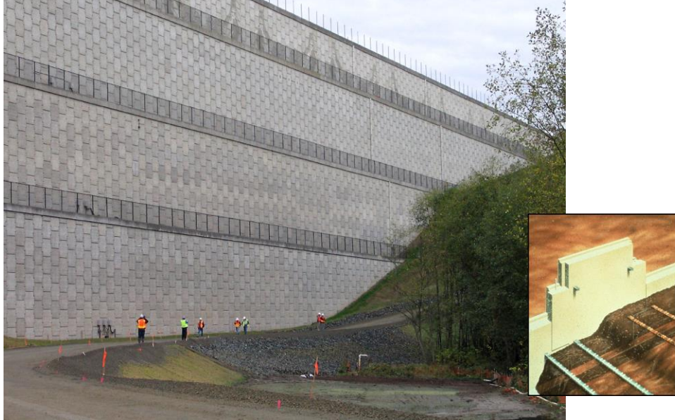
SeaTac Airport runway extension (Seattle Washington USA) - steel strip MSE wall (46 m high) (completed in 2006)
