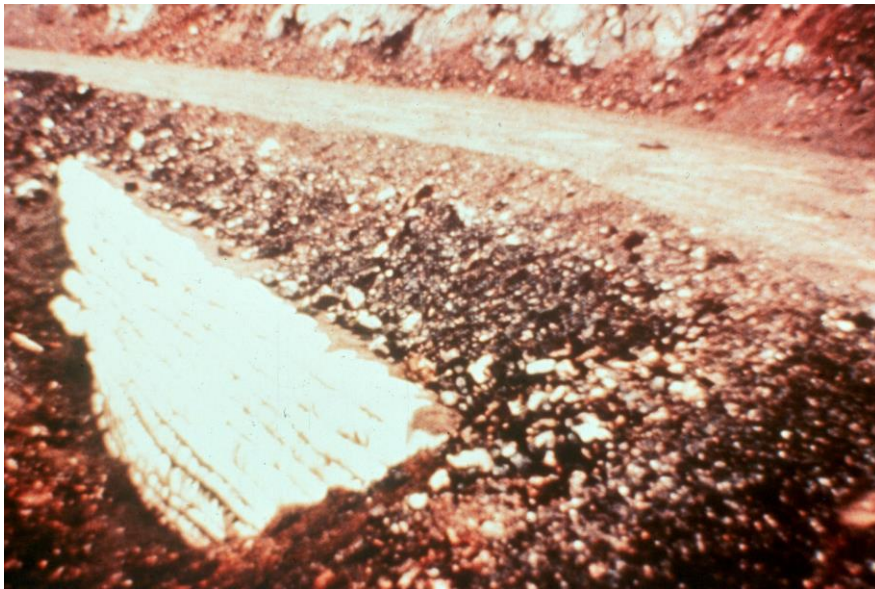
First geotextile wrapped-face wall in North America (Snailback Wall) (United States Forest Service, Oregon, 1974)
