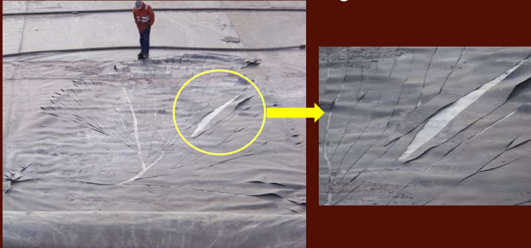
GMB stress cracking of a 1.5 mm thick HDPE geomembrane in a tailings storage facility, China in 2009 (Peggs et al .2014)
